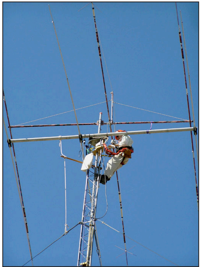
Mike Gross, KØALT's husband, connects a balun to her lowered tribander antenna during a recent tower climbing excursion.
